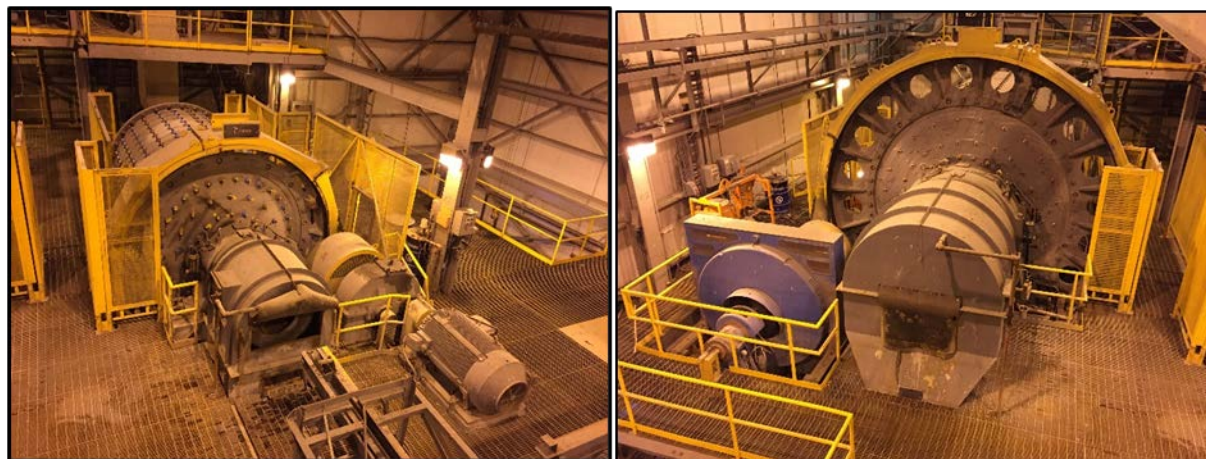
FIGURE 17.4 BUCKO PROCESS PLANT ROD AND BALL MILLS
