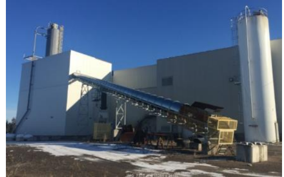
Paste Backfill Plant (2012)
