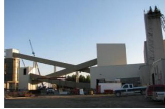
Transfer Towers & Conveyors
