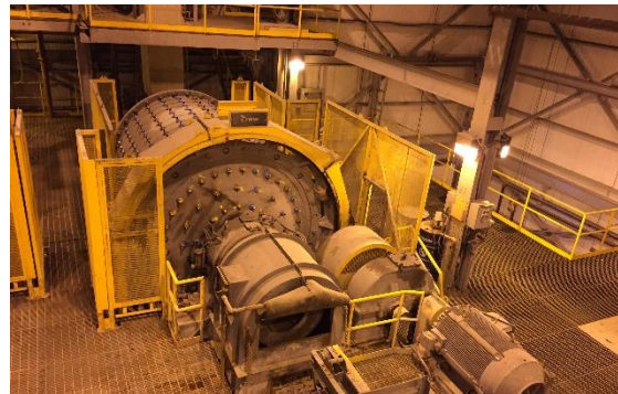
Existing Ball Mill
